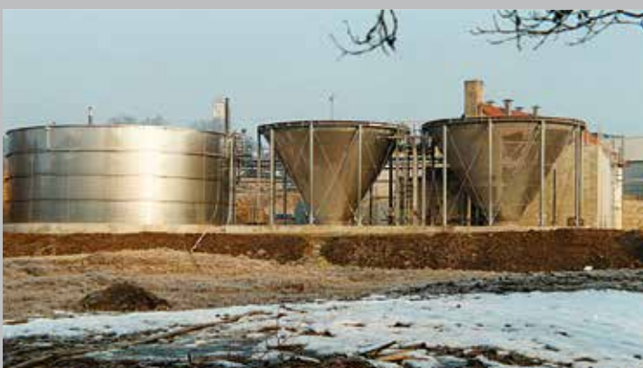
▶ Nachklärbecken ▶ Secondary sedimentation tank
